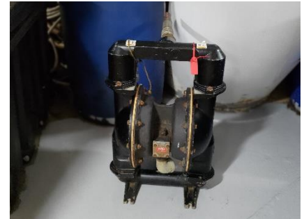
Wilden Pump no.1 for hold cleaning tagged
